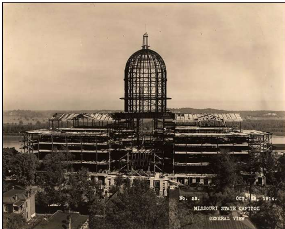
The Missouri State Capitol Building is under construction. General view looking north, October 15, 1914. (Photo from Capitol Commission RG 395 – MO Secretary of State)
